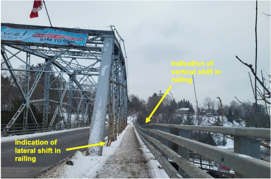
Figure 1 – Deformed barrier indicating loss of elevation
