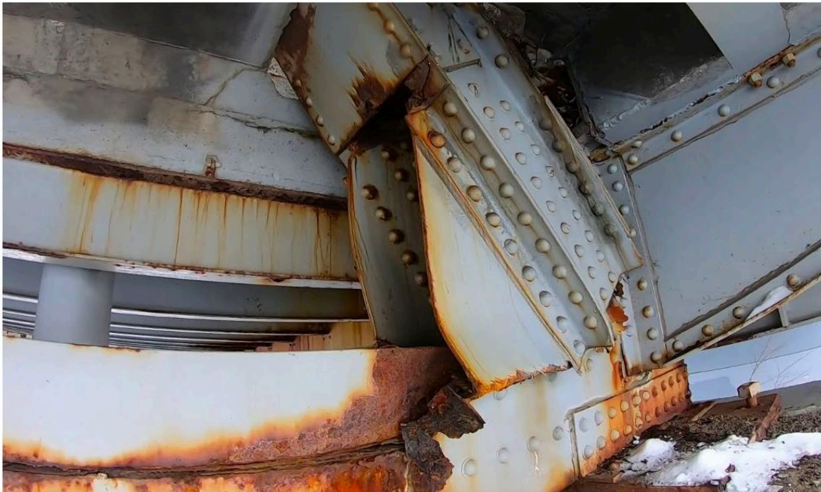
Figure 3 – Buckling of gusset plate at southwest bearing
