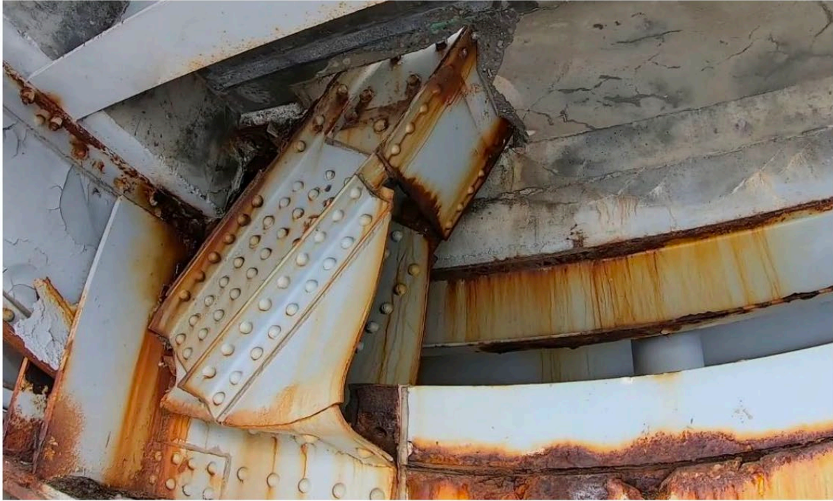
Figure 2 – Buckling of gusset plate at northwest bearing
